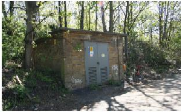
3 Existing electricity substation
